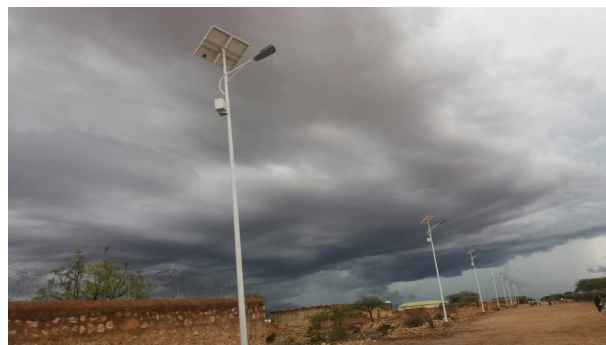
Solar Streetlights in Xudur installed during Phase II
