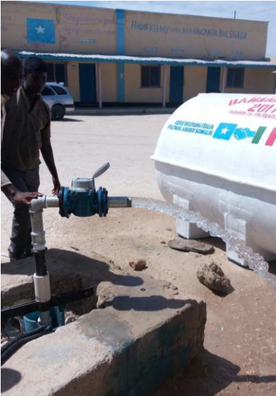
Photo 5 Solar-powered water pump
