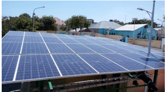
Photo 4 Newly-installed solar panels
